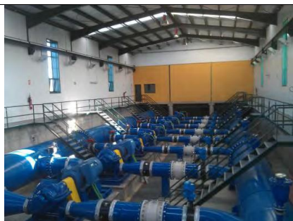
Pumping station in Porma Area
